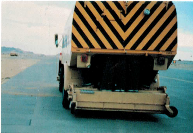
Lateral blast nozzles removing sand from runway with pickup head in retracted position.
